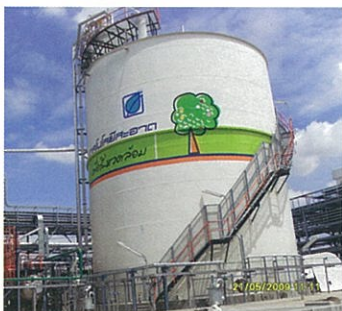
BANGCHAK PETROLEUM TANK
