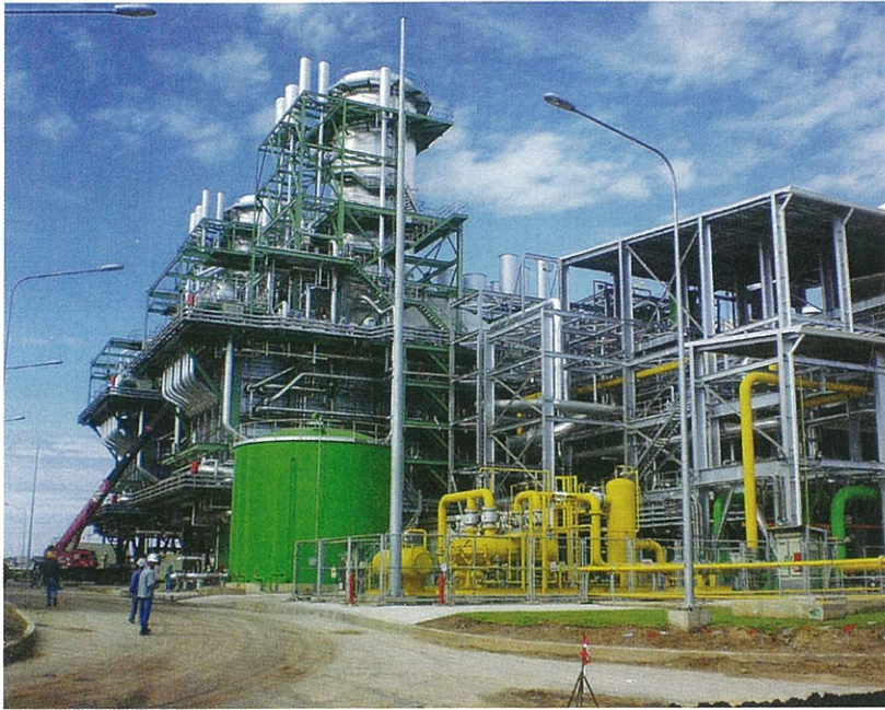
Combined cycle power plant
