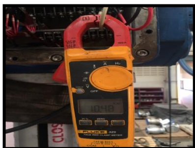
Fig 3. Current of Phase 2 (Before)
