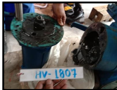
Fig 16. Inspect Motor of the Actuator
