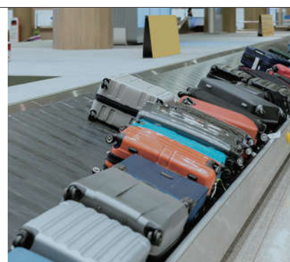
Airport baggage conveyor
