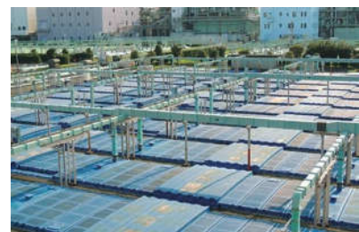
Water treatment plant
