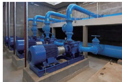
Building water pumps
