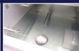
STEAM MIXER & FLOAT SWITCH
