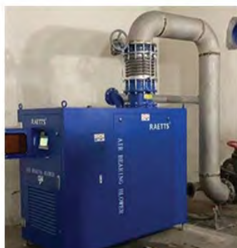
Sewage treatment factory at Guodian Galaxy
