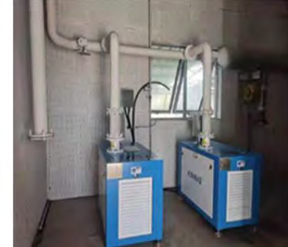
Sewage Treatment Station In Xuzhou Tongshan District
