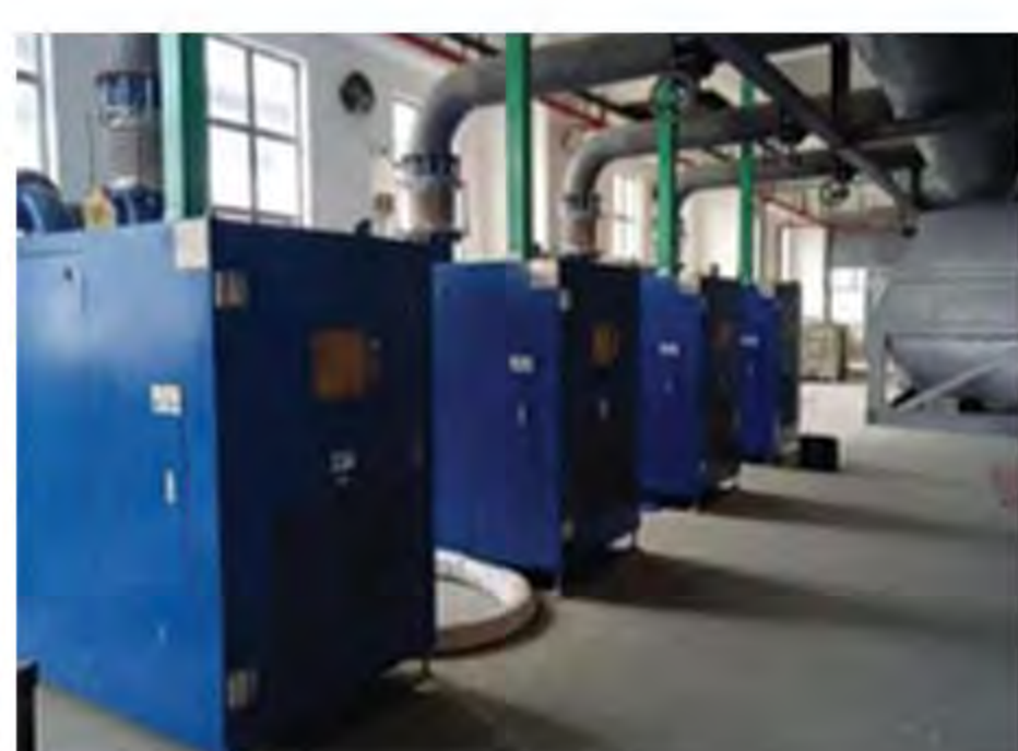
Landfill Leachate Treatment in Mayong, Dongguan
