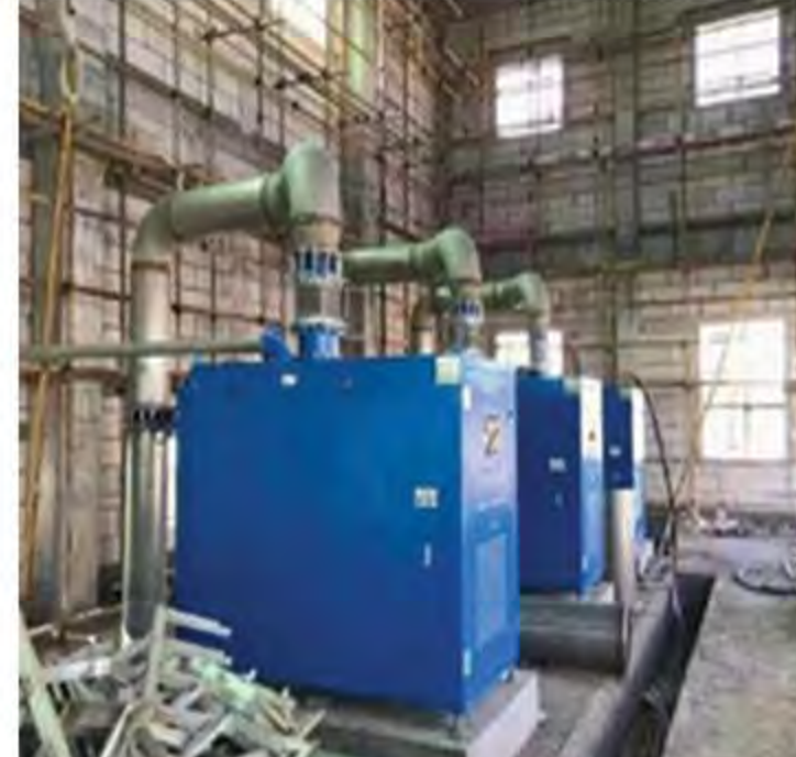
50,000 tons of sewage treatment in Anhui
