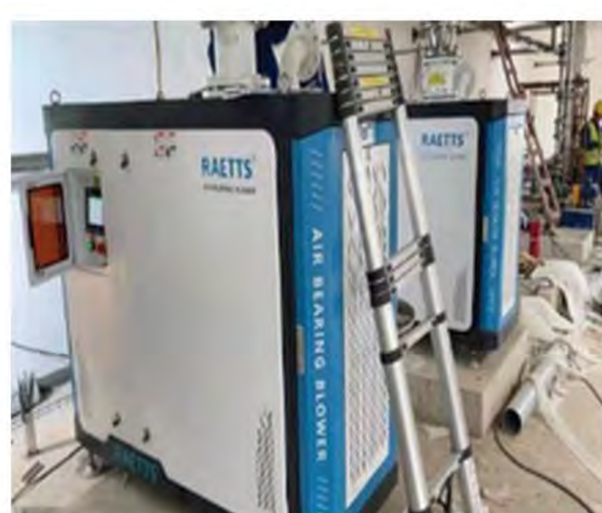
Sewage treatment factory in Guangxi
