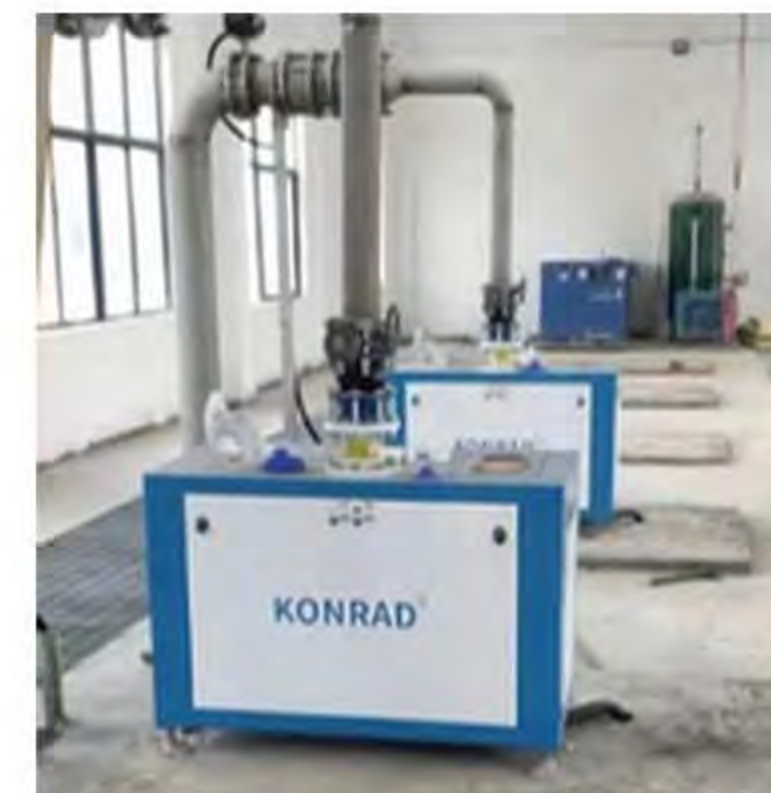
Sewage Treatment Station In Xuzhou Tongshan District
